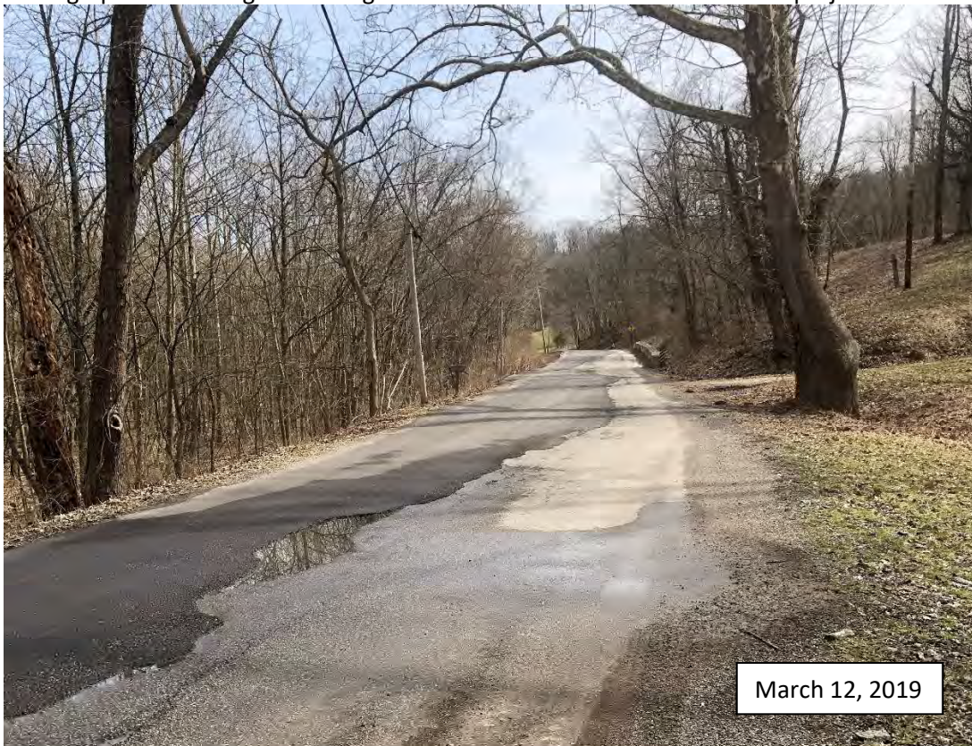
Photograph #6: Looking east along Lower Dillsboro Road near west end of project.
