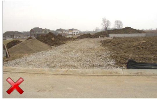
Example construction entrance at a small site. Notice the accumulation of sediment in the rock has resulting in transport onto the roadway. No diversion berm was installed to prevent sediment-laden runoff from flowing onto the roadway. Also note that the silt fence has not been properly turned uphill to prevent sediment washing onto the entrance and/or onto the public roadway.
