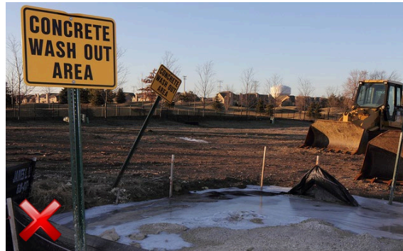
Poor job of containing washout inside of the designed area. Washout material should be removed when capacity becomes an issue.
