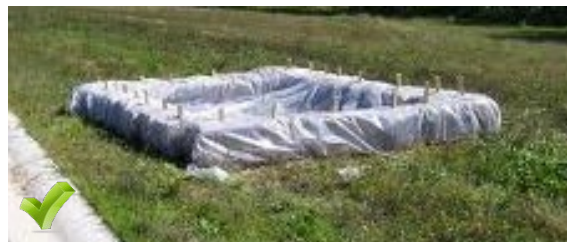
Good example of above grade system with straw bales and a polyethylene lining. A "Concrete Washout" sign should be installed at this location.
