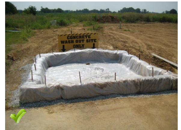
This above grade washout system has the correct polyethylene lining which is wrapped around the straw bales. The washout is underlain with DGA to provide a solid base for the washout and to prevent punctures in the plastic liner. Straw bales are securely anchored to the ground, and a large sign identifies the washout.
