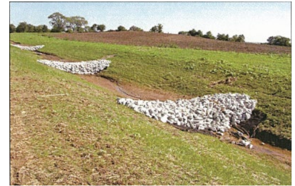
Drainage ditches need temporary silt check dams to capture sediment and reduce ditch bottom-down cutting (erosion). Check dams can be made of rock or stone-filled bags. They are only effective with smaller drainage areas, typically less than 5 acres. See table for correct check dam spacing for various channel slopes.
