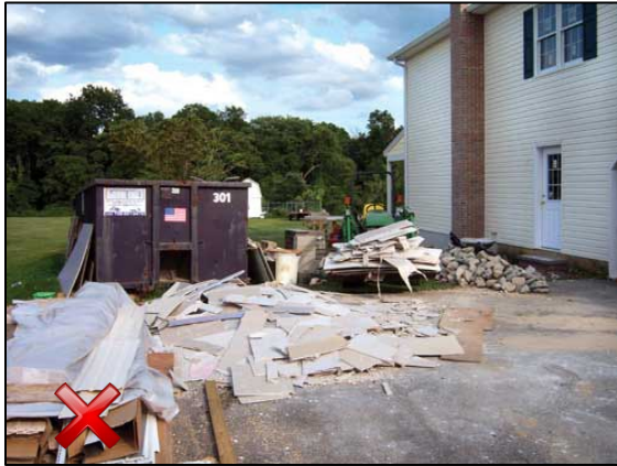
Waste material is not placed inside the dumpster allowing trash to blow around the site area and onto adjacent land. Trash is exposed to rain, which could wash pollutants into the drainage system.
