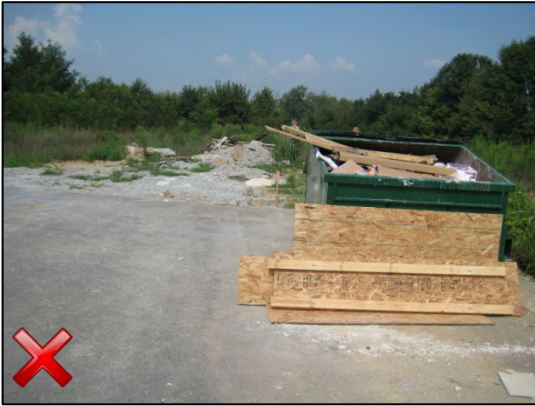
Large pieces of construction waste should be broken down and placed inside the designated disposal dumpster. Material piled up in the background should also be placed in the dumpster.
