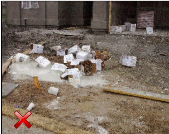
Poor trash management. Polluted runoff from the site can contaminate streams and other bodies of water.
