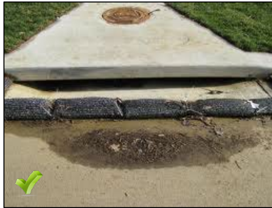
Provide inlet protection at curb inlets and/or catch basins around the building site. Never dispose of or deposit any substance into the storm collection system.
