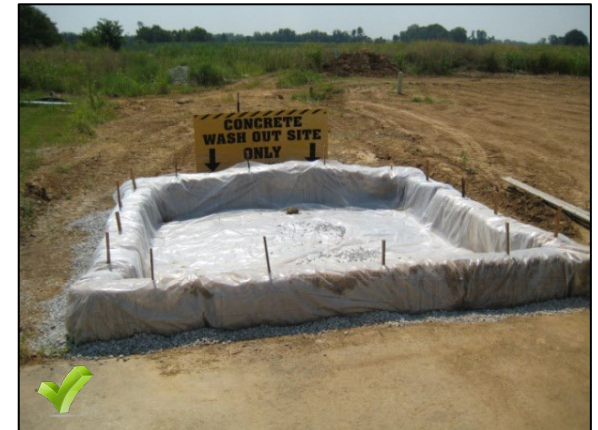
Contractors and subcontractors should utilize concrete washouts whenever pouring or placing concrete or mortar. Washouts should be used for rinsing off mortar and concrete mix, process and placement equipment. It is not acceptable to wash off equipment outside of a contained concrete washout area.
