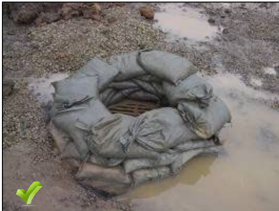
Stone-filled bags of either burlap or woven geotextile fabric should be used. Leave one bag gap in the top row to provide a spillway for overflow.
