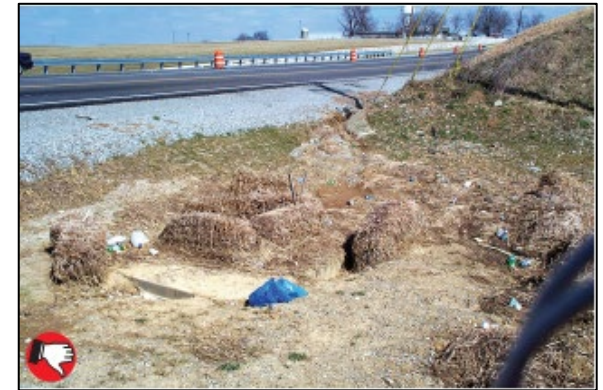
Example of poor inlet protection and inadequate maintenance.
