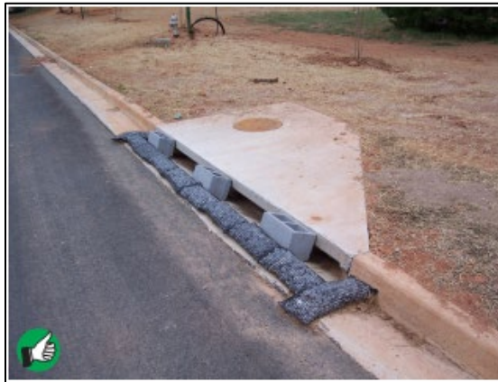
Excellent use of rock-filled mesh tubes to control sediment at curb inlet. Concrete block spacers keep tubes from moving into - and clogging - the inlet during heavy flows.
