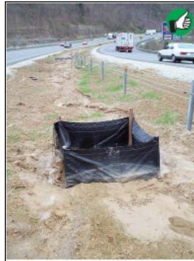
Good application of silt fence frame to protect inlet. Use wire fence backing to reinforce frame, or diagonal bracing across top of stakes. Make sure fence is trenched in to prevent bypasses or undercutting. Inspect and remove sediment as necessary after each rain. Expect a more frequent replacement schedule for silt fence drop inlet protection.
