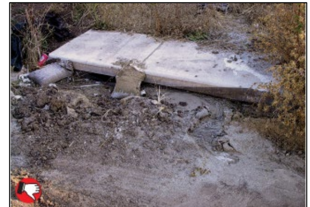
Poor placement and poor maintenance of stone bag inlet ponding dam. Accumulated sediment must be removed and dam should be repaired.
