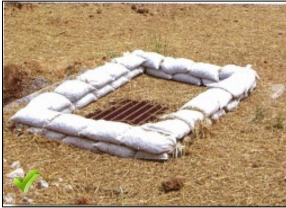
Inlet protection berm construction of half-filled stone bags. Use #57 rock, overlap bags to eliminate large openings and rapid flow-through.
