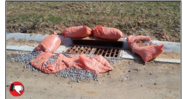
Poor placement of stone bag inlet dam. Bags work well if used properly and maintained. Bags must form a dam around the inlet with no large gaps.
