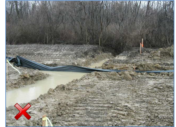
Example of poor sediment trap installation. Silt fencing should never be used as an outlet structure for a sediment trap.
