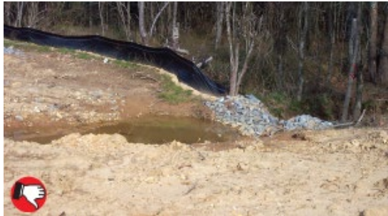
Example of poor trap installation. Overflow notch is too deep and surrounding area needs seed and mulch to prevent erosion.
