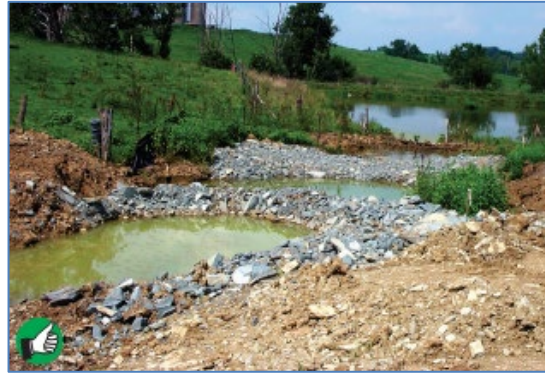
Fair installation of two traps above a small pond. Dikes are a little too small and the area needs seed and mulch.
